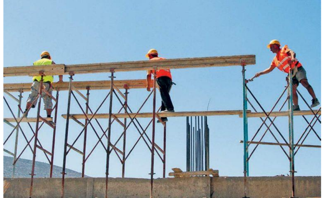
Poor health and safety measures
